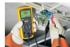
Wiring test in a small distribution box – all in one spot
