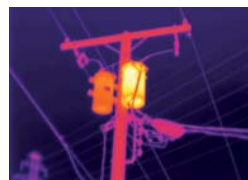
Overheating pole transformer
